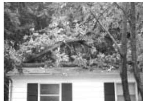
A large tree fell onto an Audubon staff residence. No one was injured.
